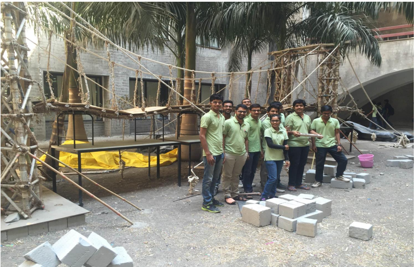
Glimpses of suspension bridge along with the team of civil engineering students.
